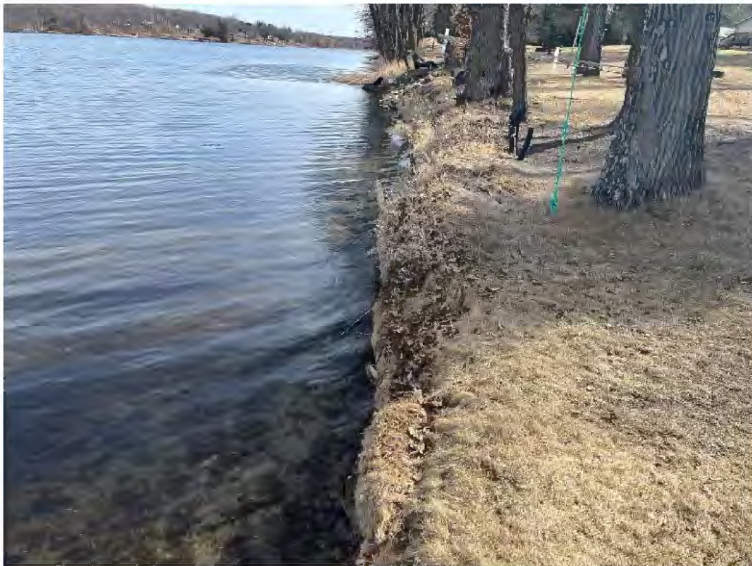
Photos from top of bank showing extent of damage to coir log
